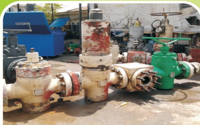
IBEWA 7 VALVE BEFORE SERVICING
