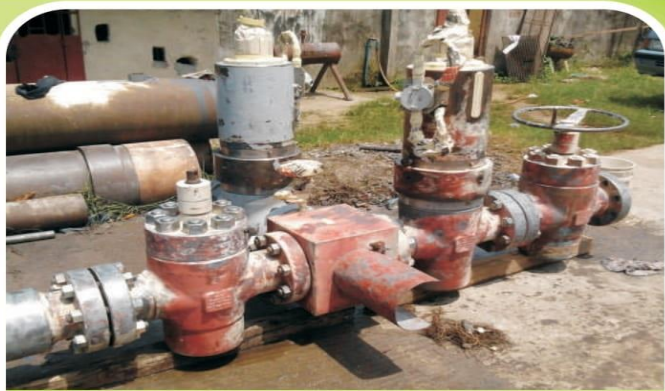
IBEWA 12 VALVE BEFORE SERVICING
