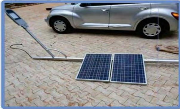
Solar Perimeter Lighting Solution at Fugar Edo State
