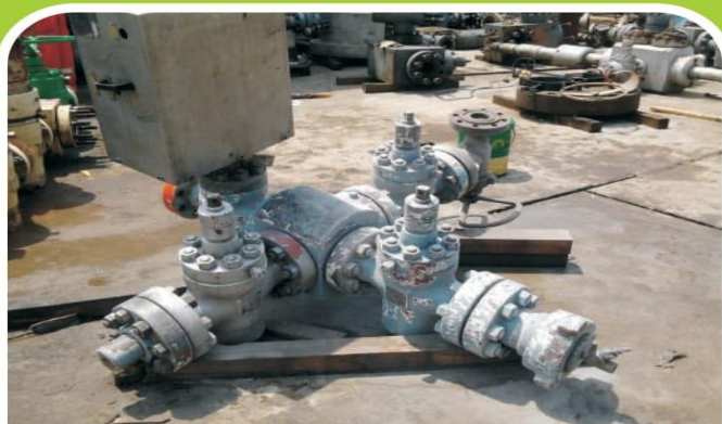
IBEWA 13 VALVE BEFORE SERVICING
